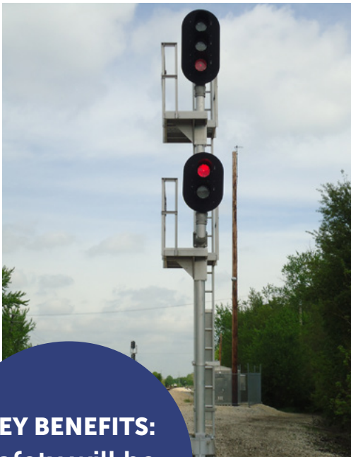
Remote controlled switch machine
