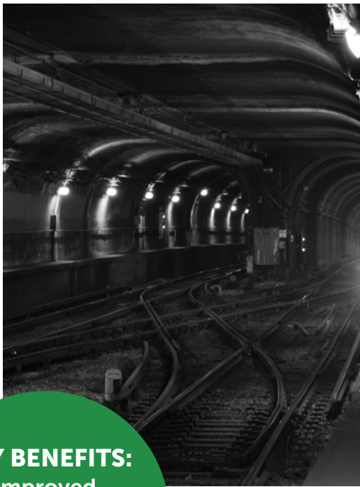
Subway ventilation improvements needed
