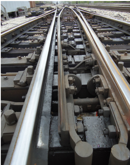
Switch components need continual care
