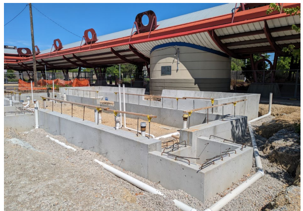
Poured foundation and underground utilities for the new ADA Transfer Center located in Schaumburg.
