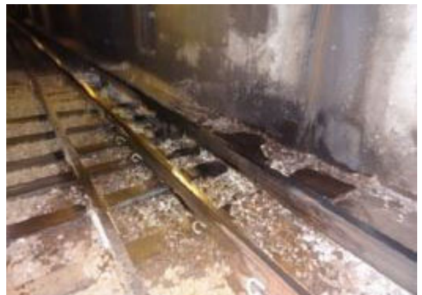
Existing water damaged area in the Kimball Subway.
